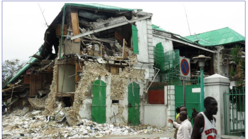
Figure 2 – Unreinforced masonry building damaged in 2010 Haiti earthquake.
